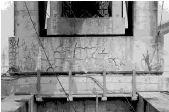
图 2 湘潭特大桥桥墩开裂形状图 Figure 2 Cracks distribution in Xiangtan bridge
